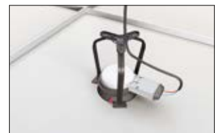
4. Connect the downlight to the power supply and fix the cable into the routing eyelet.
