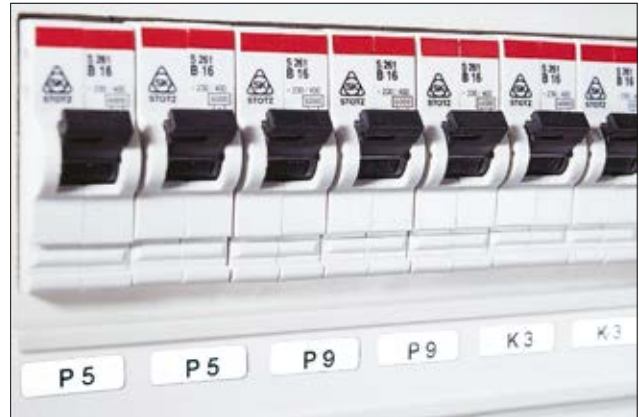
Clear and permanent identification of switch gears.
